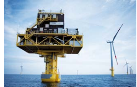
Substation OSS off EnBW wind farm Baltic 1 in the Baltic Sea Picture 1
